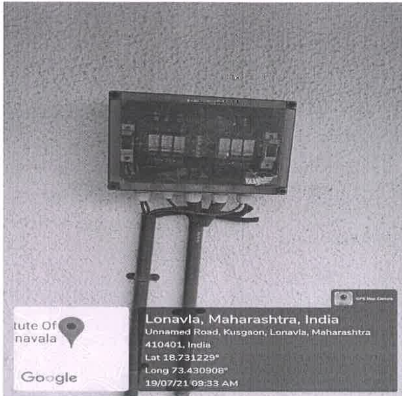
D C Distribution Board
