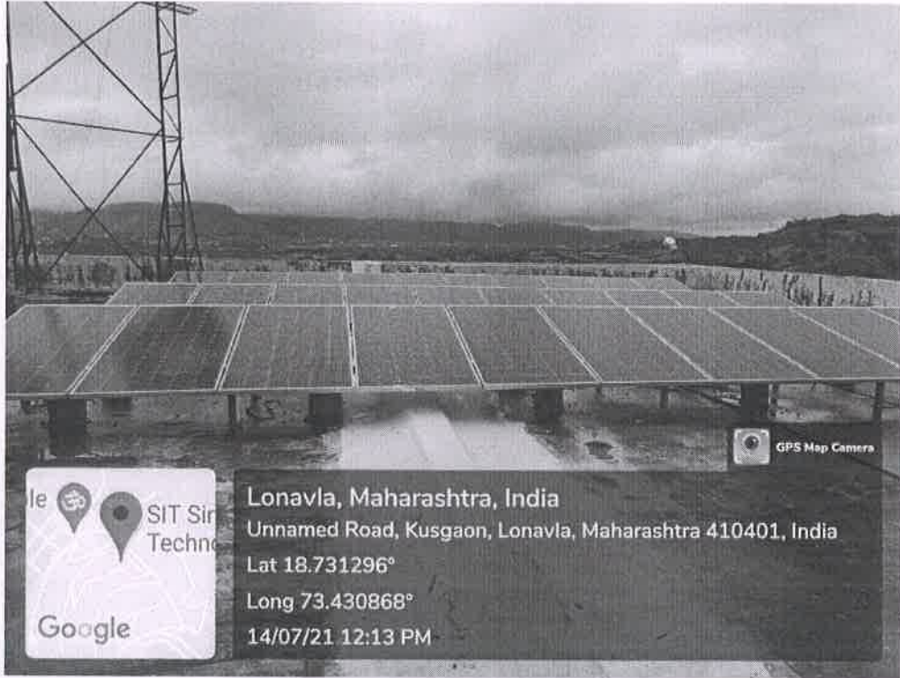
Solar Power Plant (10kW)
